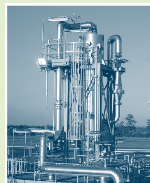
▲ The GTL plant in Chinchilla is being upgraded for its next start up, December 2009.
