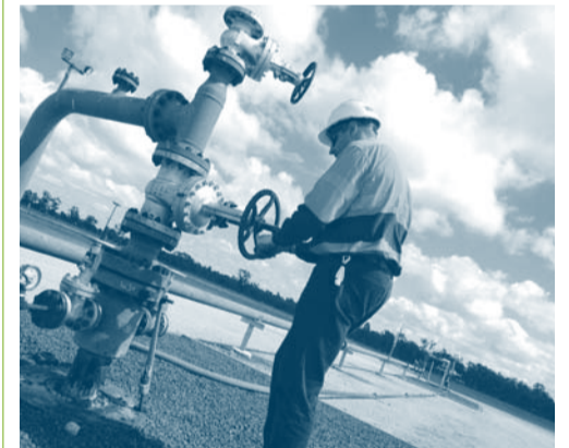
▲ Linc Energy's UCG technology leads the way for the growing UCG industry.
